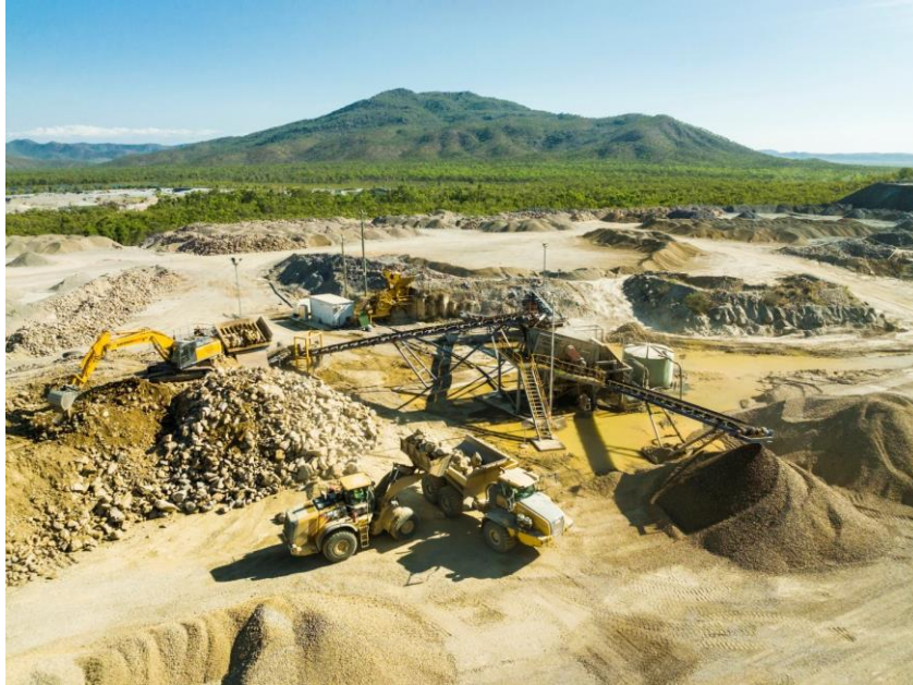
Figure 1 - Crushing plant achieving throughput targets
