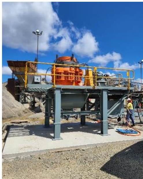
Figure 2 - Tertiary Cone Crusher for XRT Sorter Concentrate
