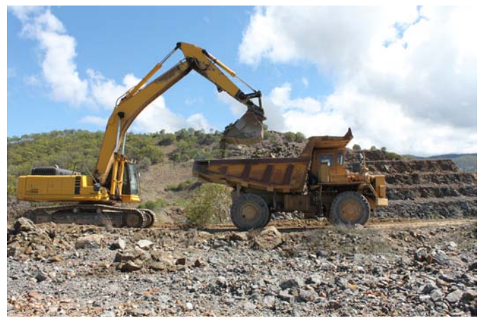
Obtaining material from the stockpiles for the testing of the X-ray ore sorter.
