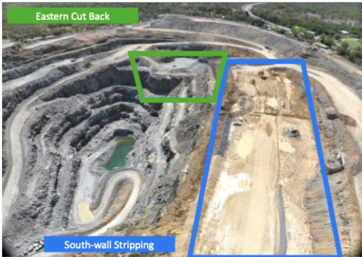
Figure 1 - Stage 2 Pit development covering the Eastern Cut Back and South-wall stripping programs
