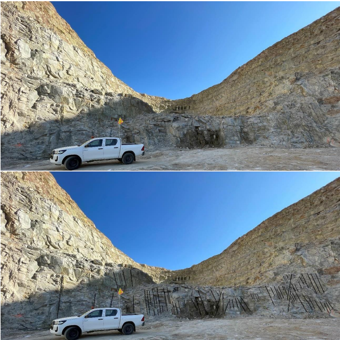
Figure 8-1 Barruecopardo northern pit wall with subvertical vein swarms and/or fractures (lower picture interpreted)
