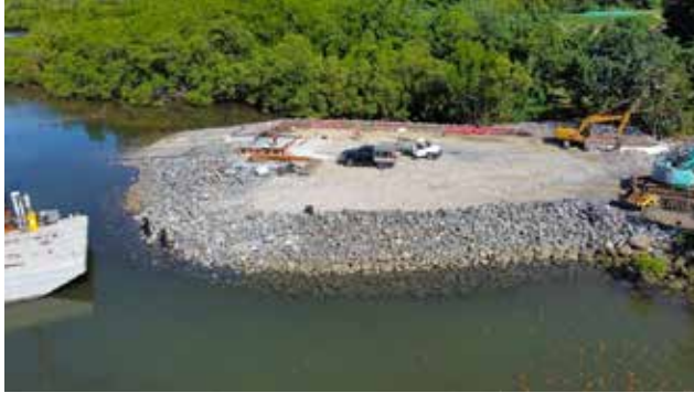
Newell Beach boat ramp newly built with Mt Carbine's green waste rock.
