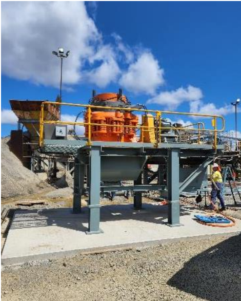
Figure 3 - Tertiary Cone Crusher for XRT Sorter concentrate
