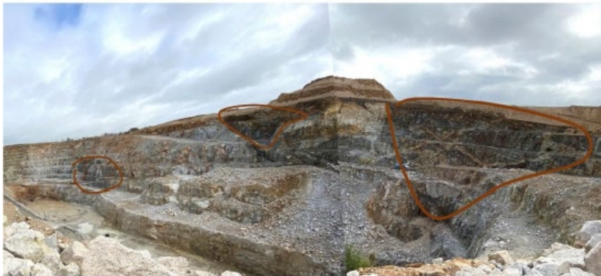
Figure 5-1 View of the east slope of the cut from the southwest, showing the areas where hornfels appear. A. Lejano. 2024
