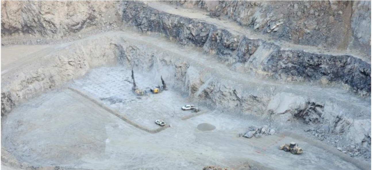
Figure 27: Orana Drill and Blast Rigs working on the holes for the first calibration blast.
