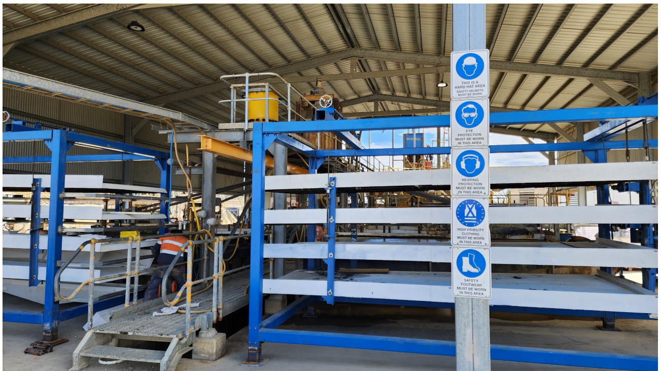
Figure 6: Eight additional shaker tables have been installed and commissioned to increase processing capacity.
