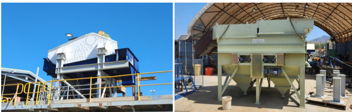
New Schenk Dewatering Screen that will be paired with the new roll crusher (Left); The new Jig being prepared for commissioning (Right)
