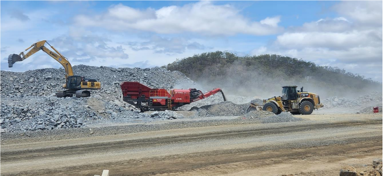
Newly commissioned Terex Finlay Jaw Crusher J-1175 with a 50 tonnes excavator and a CAT 980M preparing the feed on ROM1 Stockpile for the Crushing Plant
