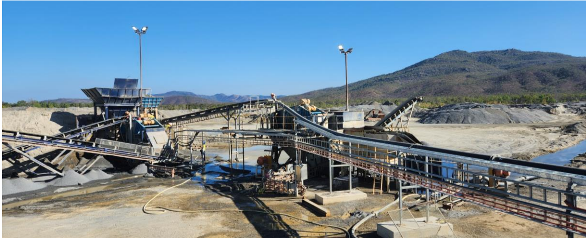
The High-Grade Crushing Circuit on the left, vibrating screen and new Jig on the right, the 6mm fines pipeline at the foreground, pumping fines from the crushing plant straight to the screen.
