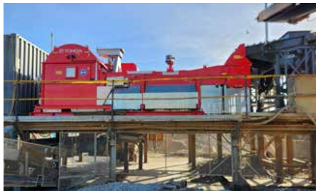
Newly commissioned TOMRA 3 Ore Sorter.
