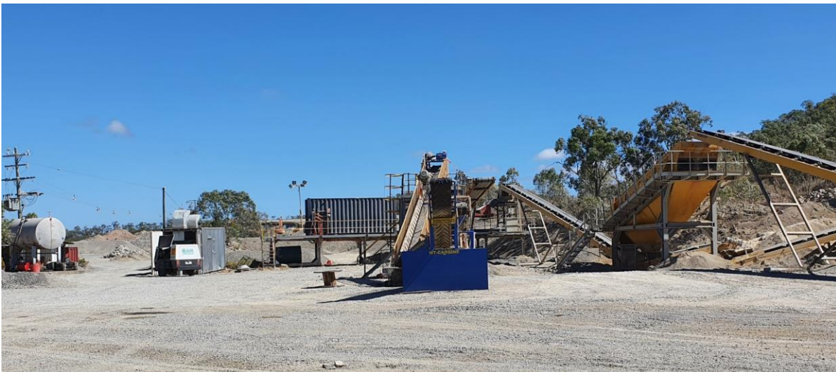
Figure 26: Existing Ore Sorter
