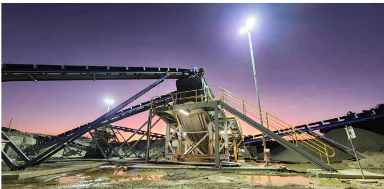
The Crushing Plant at dusk at Mt Carbine with its vibrating screen in the foreground and cone crusher in the background.
