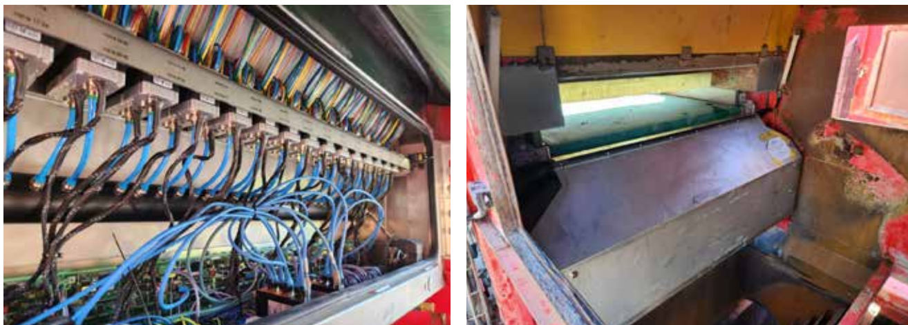
Inside TOMRA Ore Sorter #2 showing the valve bank (left) and the end of the conveyor belt where the material gets ejected (right).
