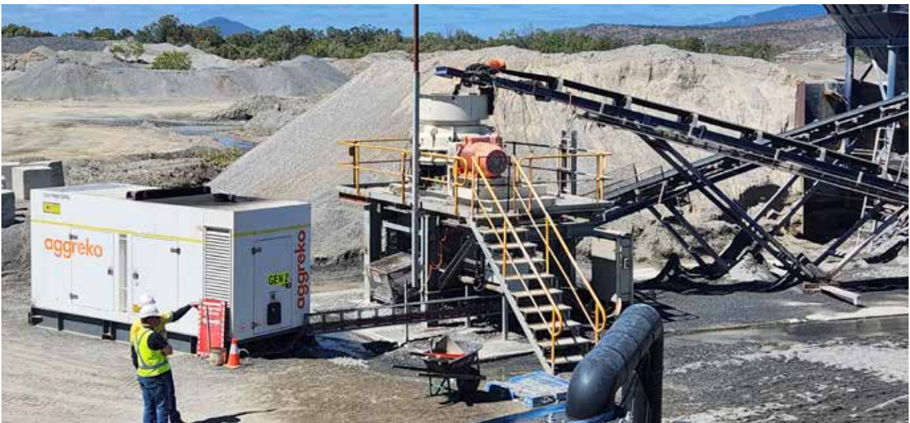
The High-Grade Crushing Circuit at the Gravity Plant.
