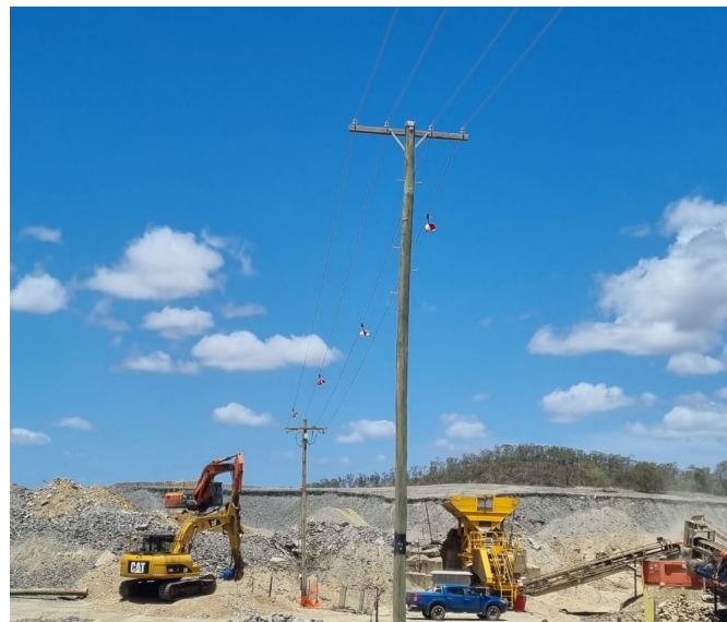
Fig.1 – Extended power line dedicated for increased XRT Sorter production.
