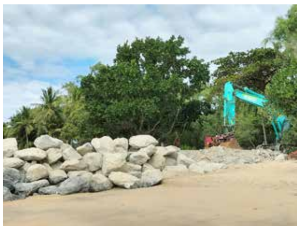
Mt Carbine Quarry armor rock used on the Cairns Northern Beaches for boat ramps, beach protection and jetty.
