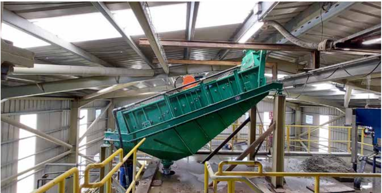
Picture above: The Multideck Screen being commissioned.
