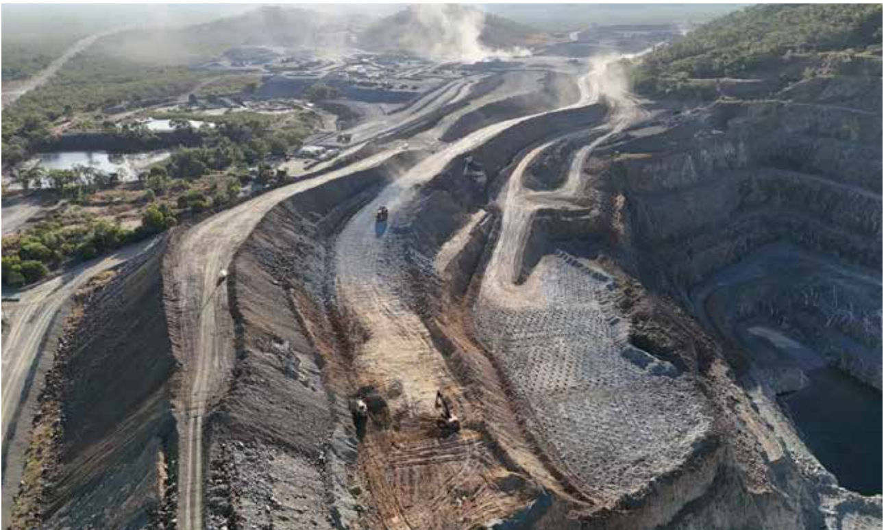
Picture above: Stripping activities progressing in the South side of the open pit where the old crushing plant used to stand.
